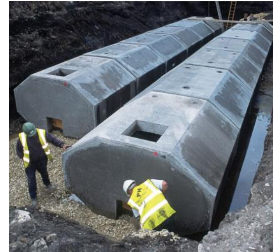
Photo – Pre-cast concrete storage units
