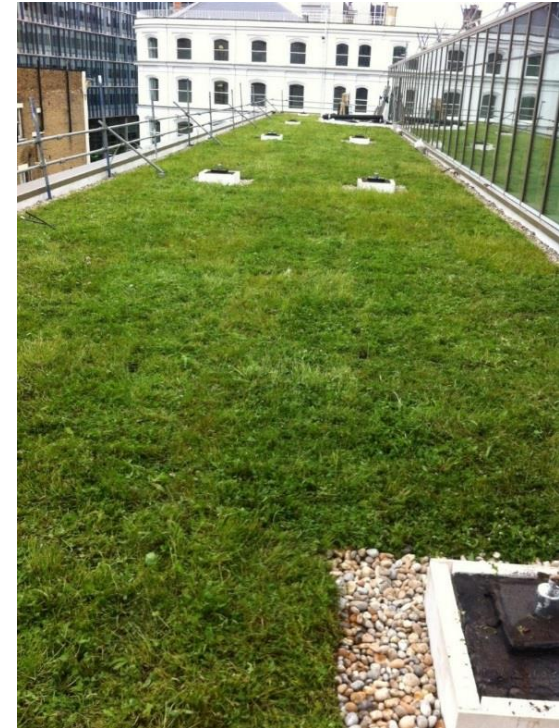
Photo – Extensive green roof
